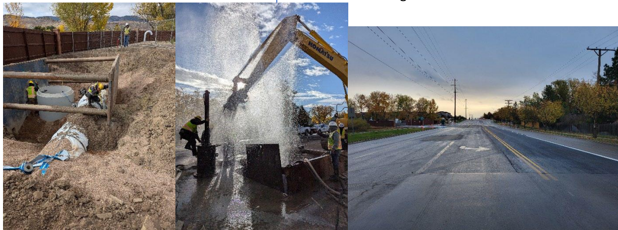
Left: 42" Butterfly Valve Vault
