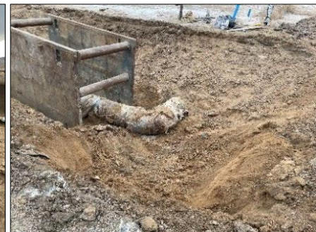
Right: Existing 24” 90 degree bend and tie in location for the 30” feeder pipe line to the existing 4 MG Tank
