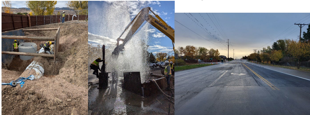
Left: 42" Butterfly Valve Vault Center: Line stop removal Right: Final pavement and striping
