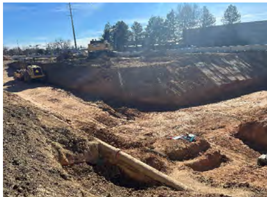
Above: Showing a section of our existing 10" AC waterline in conflict with the project excavation
