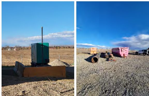
Left: Generator protected from demolition activities Right: Site piping removed from existing pump station
