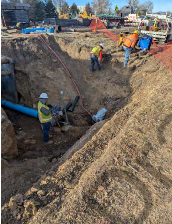
Above: New segment of waterline awaiting connection to our existing 10" AC line.
